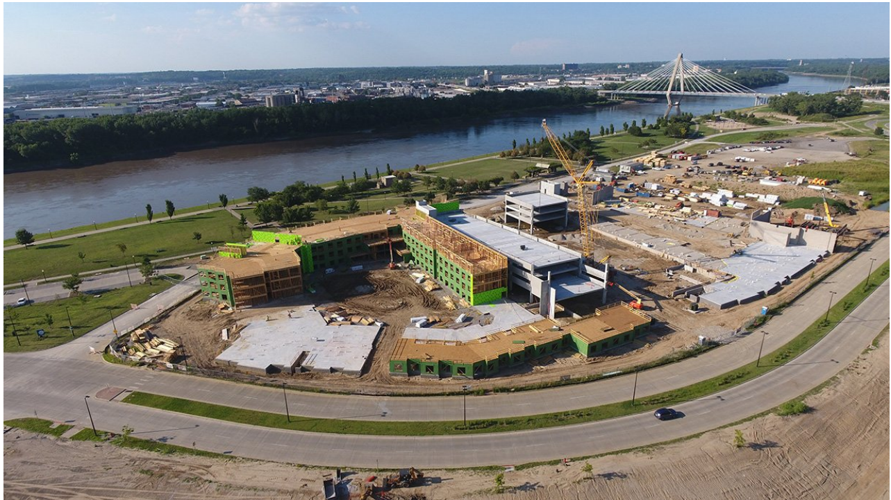
Figure 41 Looking in a northerly direction at the Flaherty and Collins construction on the riverfront (July 2017).
