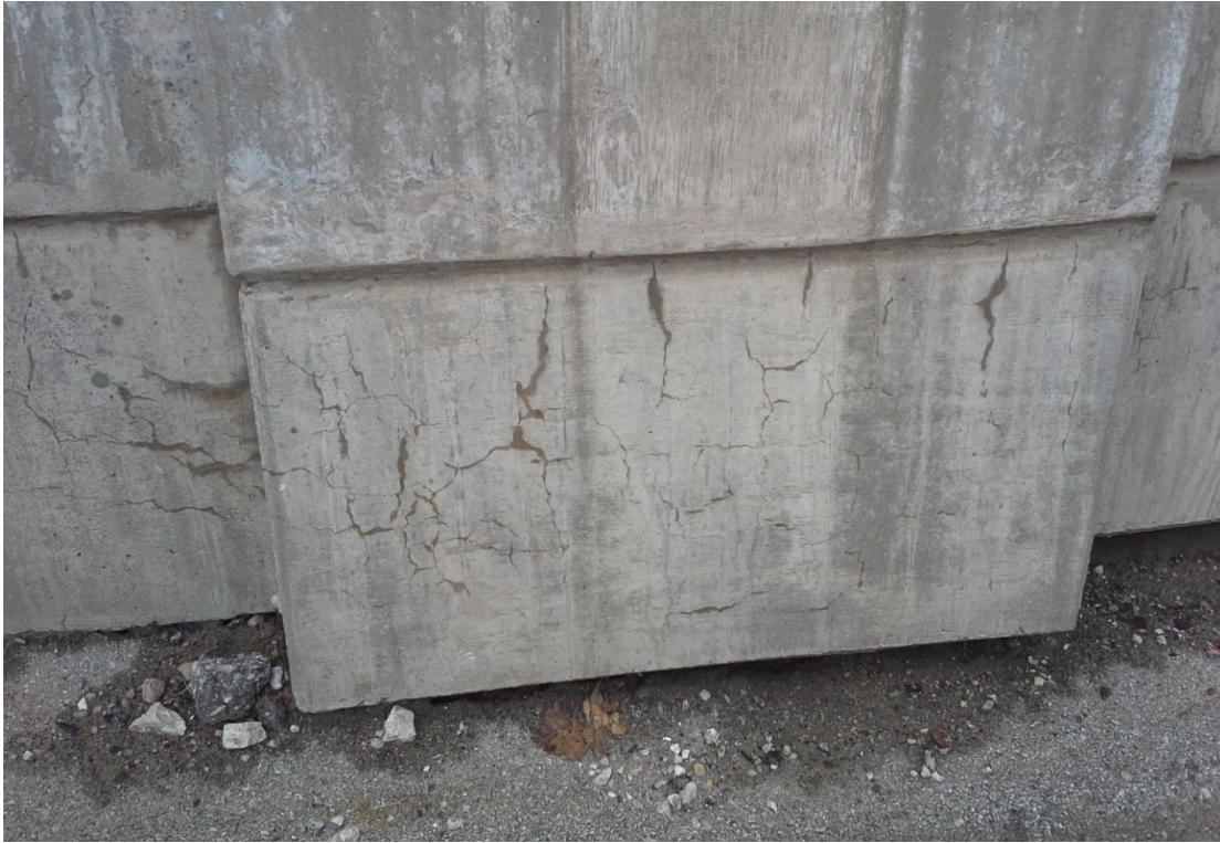
Figure 55 Cracks in Base of Barrier Post on MSE Wall Segment
