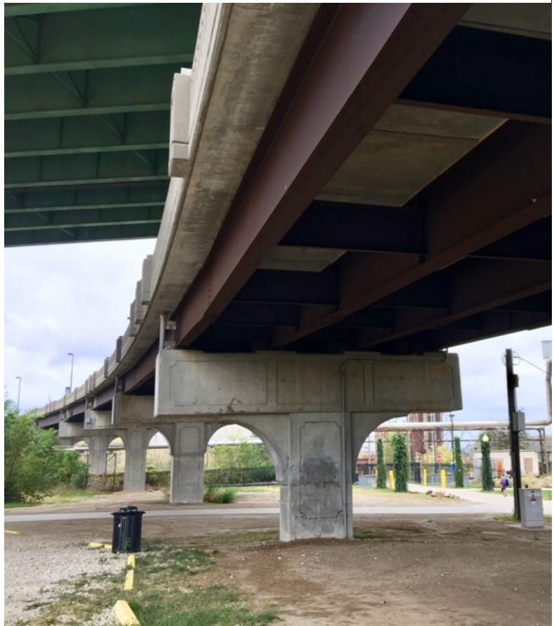
Figure 9 View of Grand Ave Bridge under the Heart of America Bridge taken from Riverfront elevation.
