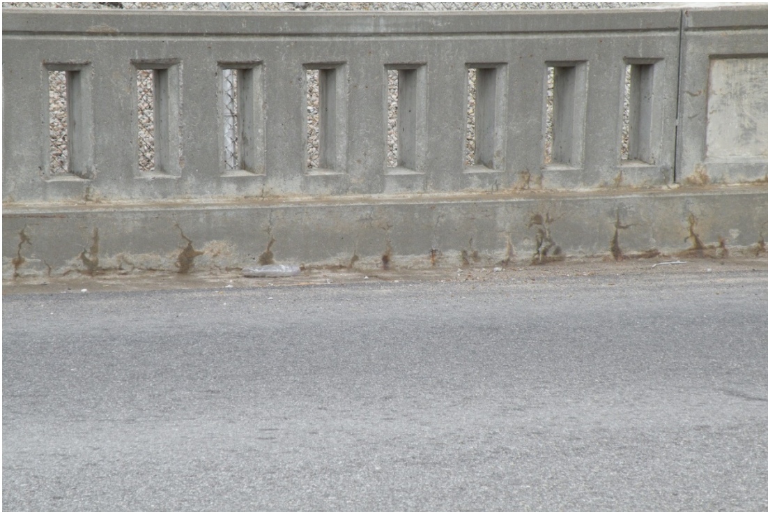
Figure 54 Cathedral Barrier Wall and Crack in West Curb on MSE Wall Segment
